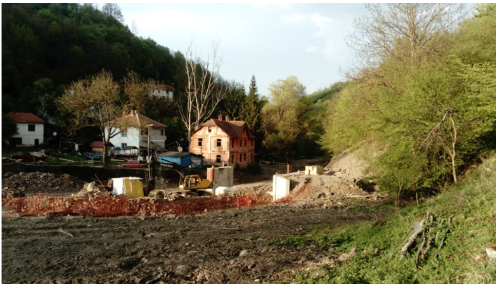
Construction of hydropower plant in the middle of Rakita on the Rakitska River. Photo: Iva Marković
